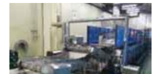
Water Tank Cooling (Installed coolers) ▶
